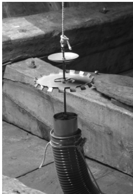
Fig. 6. Specially designed duct heads used to provide efficient distribution of climatized air inside the ship. Photograph by the author.
